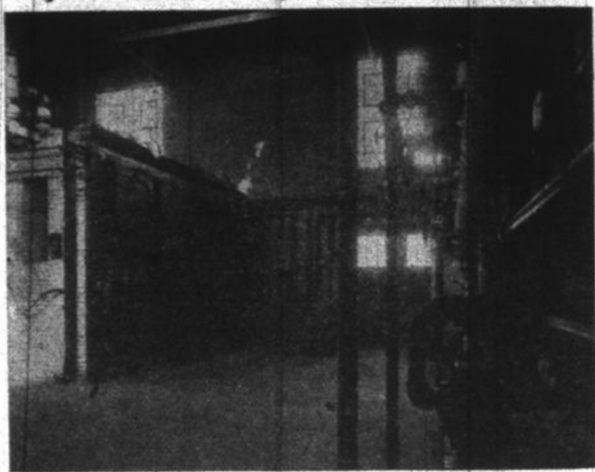
FIG. 2. GENERAL VIEW OF BOILER ROOM
