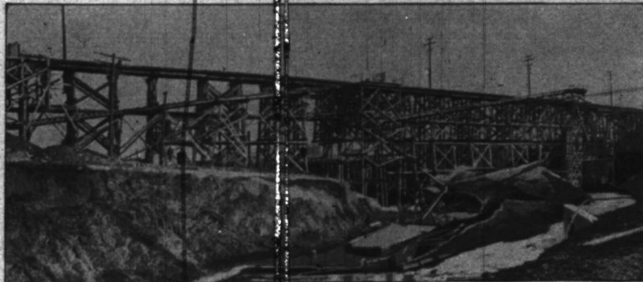
November 21st, 1917. Showing the work on the concrete trestle over the Kinnickinnick River practically completed.
