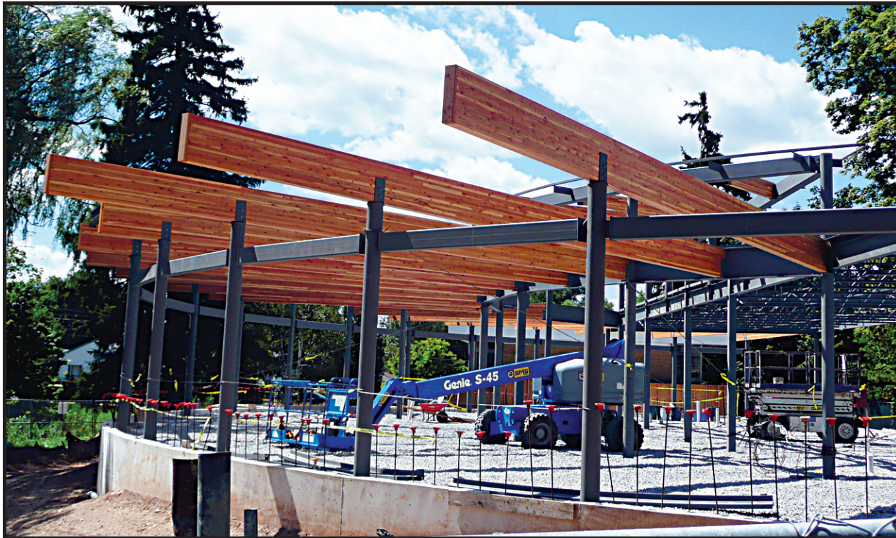
LIKE THE GLULAM? Beams made with glulam – glued laminated timber – have been installed at the River Street site of the new library. They will be visible both inside and outside the facility. – Frances Niblock photo
