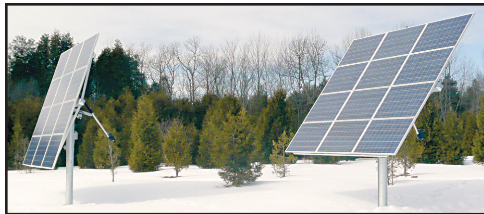
SOLAR SYSTEM: Four solar panels installed in the backyard of a Crewson's Corners residence are putting electricity into the grid and making the homeowner money – part of a provincial program to jump-start Ontario's alternative energy program by providing stable, guaranteed pricing to renewable energy producers of all sizes. – Frances Niblock photo
