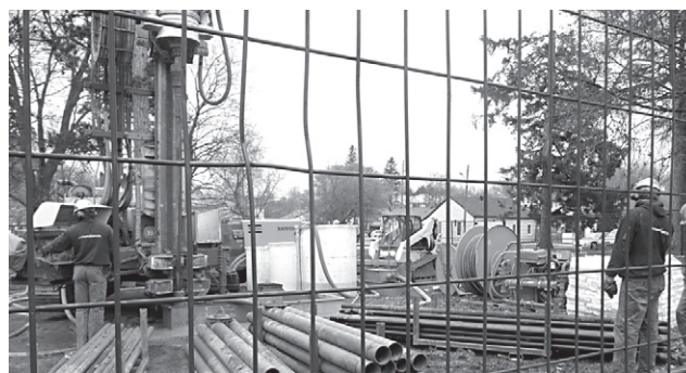
GEOHERMAL TESTING: Temperature testing 500 feet underground determined if a geothermal heating/cooling system would work at the new Acton library.
