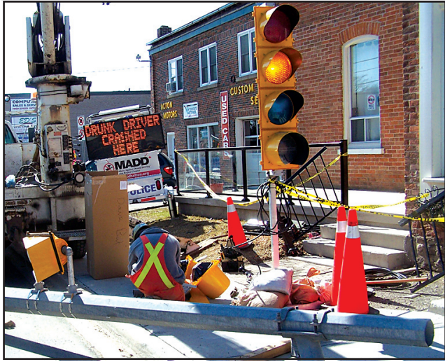
THE SIGN SAYS IT ALL: Stacey Electric was busy last Thursday fixing the light pole at Mill and Main Sts., after a drunk driver lost control and took out the pole and the railings for the building on the corner. Police posted their electronic road side sign indicating that this was the scene of a drunk driving accident at the scene of the crash which occurred on Saturday March 28 - Marie Shadbolt Photo
