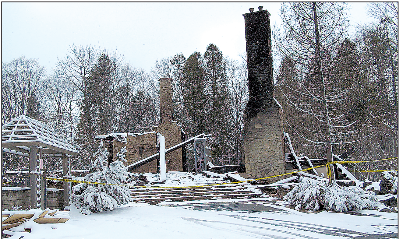
CHARRED REMAINS: This $1.1 million century-old log home undersontruction on 27 sideroad at Silvercreek was levelled by a suspicious fire early Saturday morning. Halton Detective Colin Grierson said the cause of the fire remains undetermined at this point - Marie Shadbolt photo
