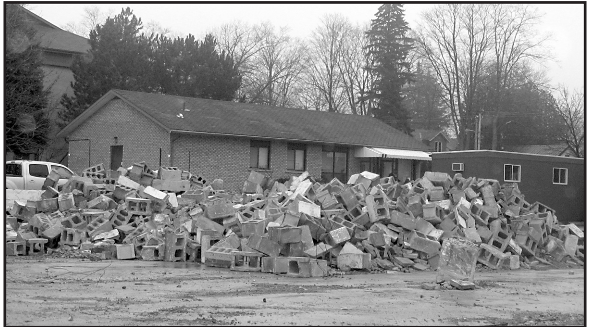
MAKING ROOM: The old fire hall in Rockwood was demolished this week to clear the way for construction of a new medical centre on the property, which will begin soon. - Rebecca Ring Photo
