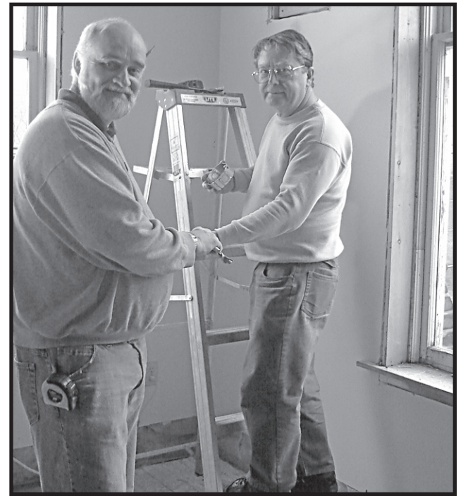
RESTORATION: Ron Birrell and Bill Sanford, along with several other Heritage Acton volunteers, spent last Saturday continuing to work on restoring the historic Acton Town Hall on Willow Street so it can again be a centre for a variety of community events. - submitted photo
