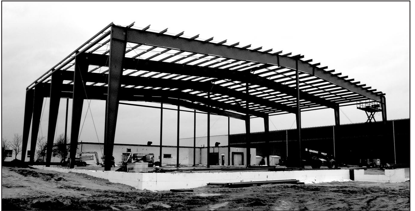
NEW BUILDING: Superior Glove begins the construction of its new building, an expansion that will not only increase business but also be power efficient. This skeleton is the first stage of the building, which can be seen from Hwy 25. Completion date is set for March 10. - Justina Pembleton photo.
