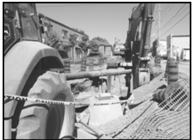
Reconstruction of Main St. from Kingham Rd. to Knox Ave. started in August
