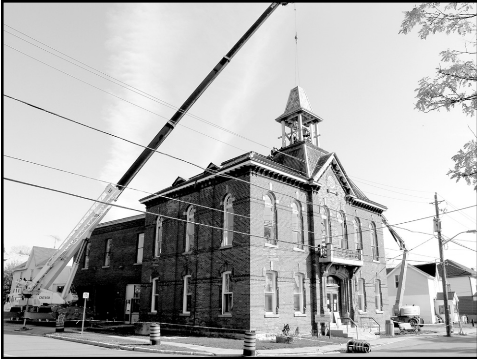
NEW CROWN: A large crane moves the new tower to its seat on the old town hall. - Ted Tyler photo
