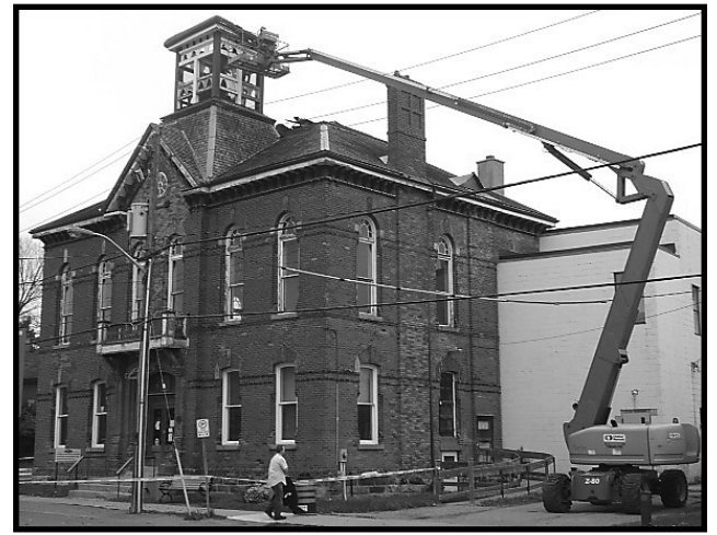
REMOVING TOWER: Renovations to rebuild the old Town Hall's roof and bell tower started on Thursday, Oct. 25 with removal of the tower. — Matthew Reid photo
