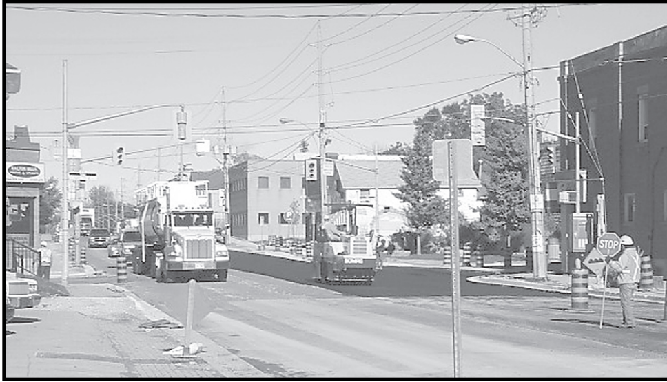
FINISHING TOUCHES: The construction along Main Street from Superior Glove north past Mill Street will be completed by this weekend. - Matt Reid photo
