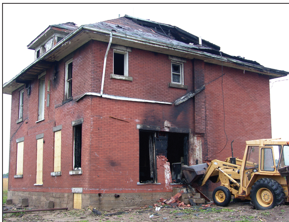
HOUSE FIRE: Firefighters from Acton were called to this home on Hwy 7, east of Acton to quench a fire. The home was being renovated for a proposed golf course. - Angela Tyler photo.
