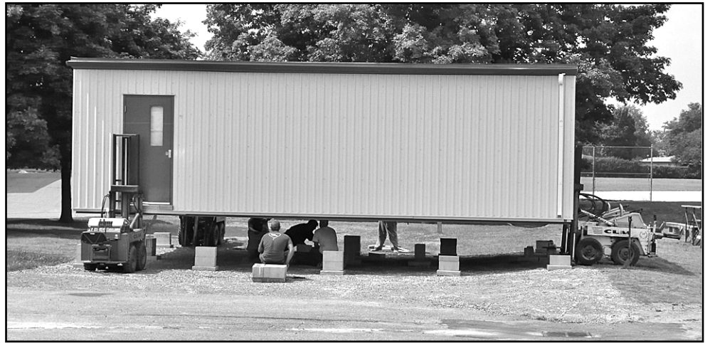
PORTABLES PLACED: Crews moved two portable classrooms onto the grounds of McKenzie-Smith Bennett School last Thursday, ready for the projected enrolment of approximately 670 students in September, up from 660 this past school year. — Frances Niblock photo
