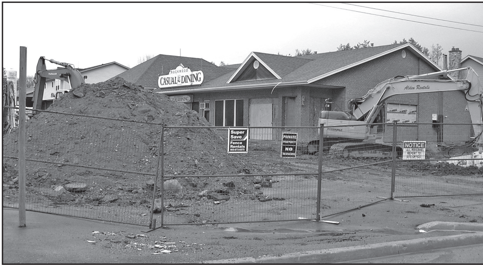
GASSING UP: Construction began on the renovations at the gas station at Fall and Alma Streets in Rockwood. Owner Dave Jassal says it will be a Petro Canada with three islands, a state of the art convenience store with movie, gift and card sections, and a Country Style Coffee Shop. The neighbouring restaurant and bar will remain open during construction. Jassal hopes to open in early May. Rebecca Ring Photo
