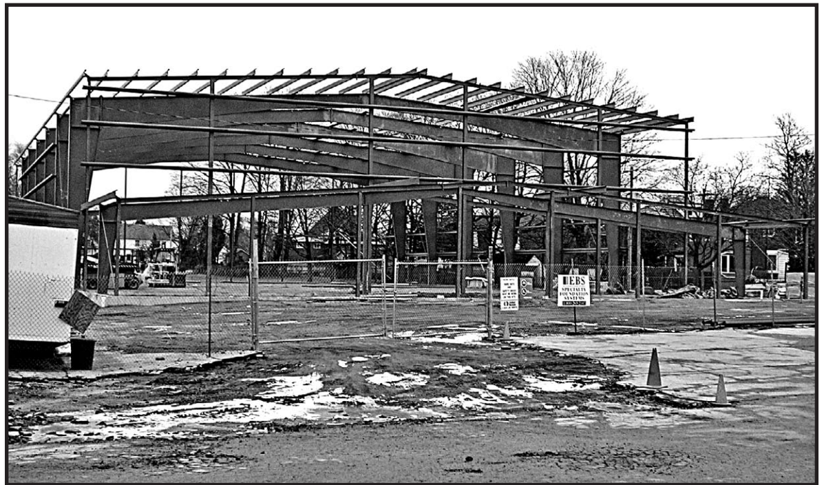
GOIN' UP: Structural steel for the new Acton Agricultural Society's building in Prospect Park is all in place and Tambro CONstruction, general contractors, are starting work on the cladding and concrete block facing. Completion of the building is targeted for late spring but the fine weather this area has been enjoying may speed completion up.
