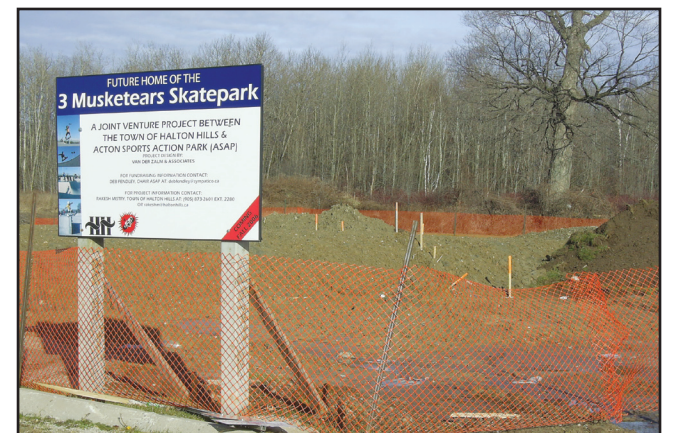
BOARDERS BUMMER: Wet weather has stalled work at the Three Musketeers Skatepark on Tanners Drive. Construction has been halted and the completion date pushed to June.— Frances Niblock photo
