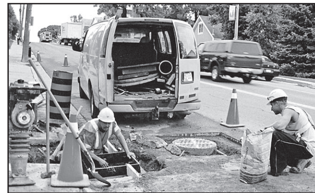
HAZARDOUS MANHOLE: Workers hired by the MTO were repairing a dangerous raised manhole on Main St. S. that is believed to have caused at least three serious cycling accidents. - Rebecca Ring Photo
