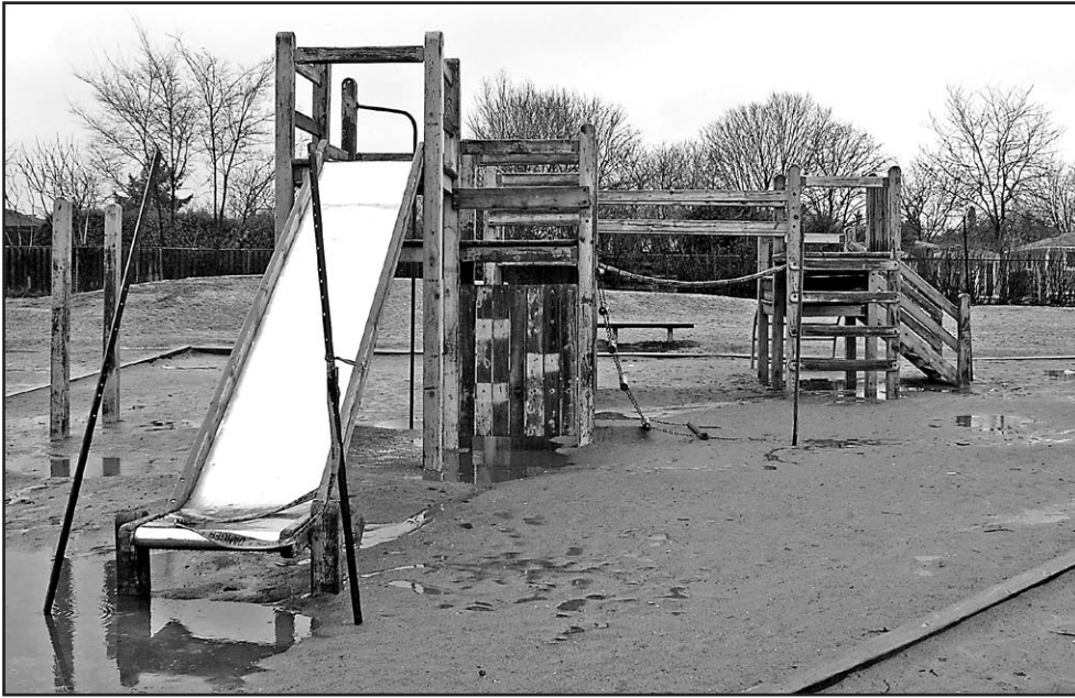
UNSAFE PLAYGROUND: A recent inspection found that the playground equipment at McKenzie-Smith Bennett School was unsafe and of "limited play value." It was slated for removal yesterday (Wednesday). — Frances Niblock photo
