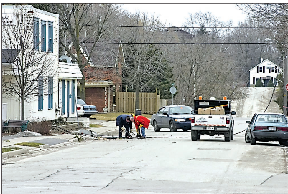
SPARK SHOOTER: Halton Police and Halton Hills Hydro shut down Church St. on Wednesday morning after hydro wires were pulled down and the meter yanked off Blue Springs Funeral Home. Power was out for several hours. - Submitted photo
