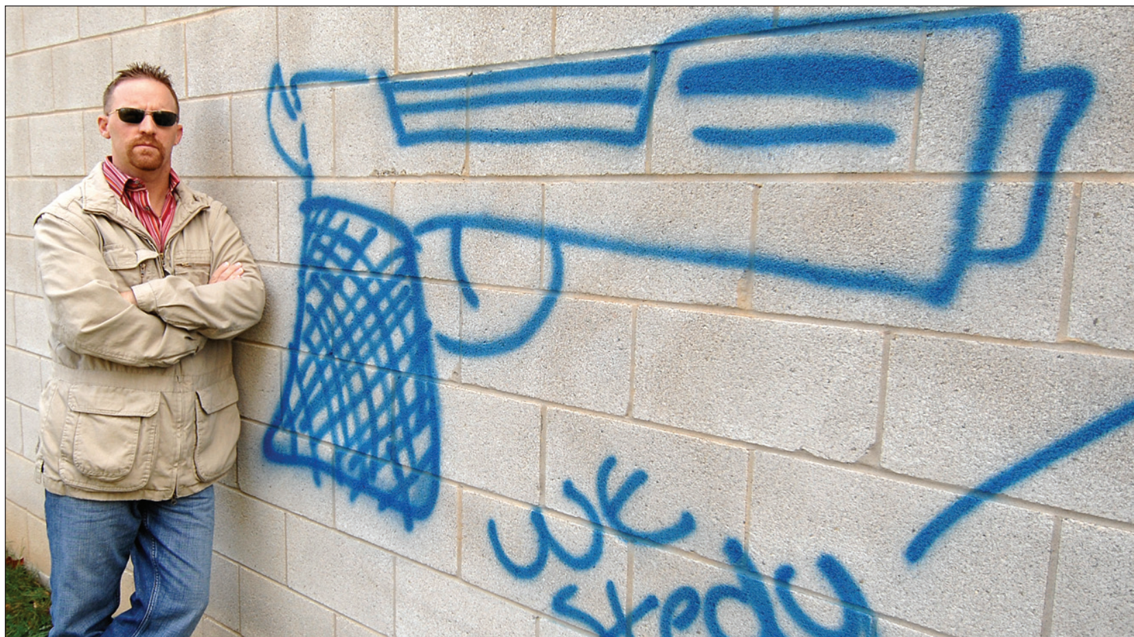
Michael Jander of Acton stands beside some graffiti which was recently painted on the side of St. George's Anglican Church in Georgetown. Jander, the owner of CAMA International, has developed a graffiti eradication program and is hoping local businesses will contribute to the plan which has the backing of the Town of Halton Hills. Photo by Ted Brown
