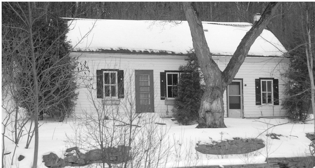
Halton Hills council has given family members associated with Beecham House, a mid-19th Century farmhouse located on 27 Sideroad, six months to find a way to salvage the homestead. Credit Valley Conservation wants to deconstruct the house saying it is a target for vandals and a safety hazard. Relatives of the home's previous owners contend the CVC let it fall into disrepair. Photo by Ted Brown
