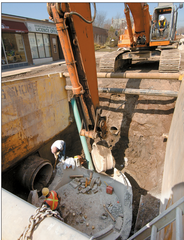
Work is progressing on Main Street in downtown Georgetown with Aecon Contracting replacing the three maintenance holes. Photo by Ted Brown
