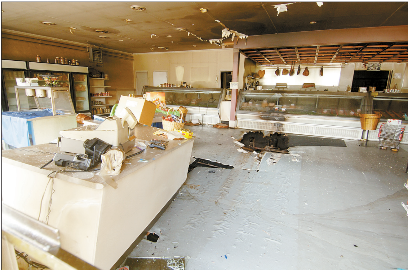
A fire at Agram Meats on Trafalgar Road in Stewarttown caused an estimated $250,000 damage according to Halton Hills fire department officials. The blaze was spotted at 4:30 a.m. Thursday by a patrolling Halton Police officer. Photo by Ted Brown
