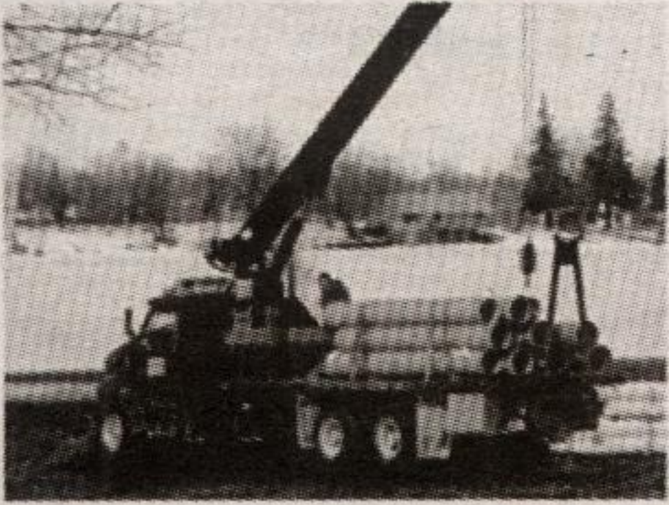
Water found! Workers bring in the Not-So-Big Pipe to Acton's Fairy Lake. The lake is expected to supply the town with water in an effort to speed up development.
