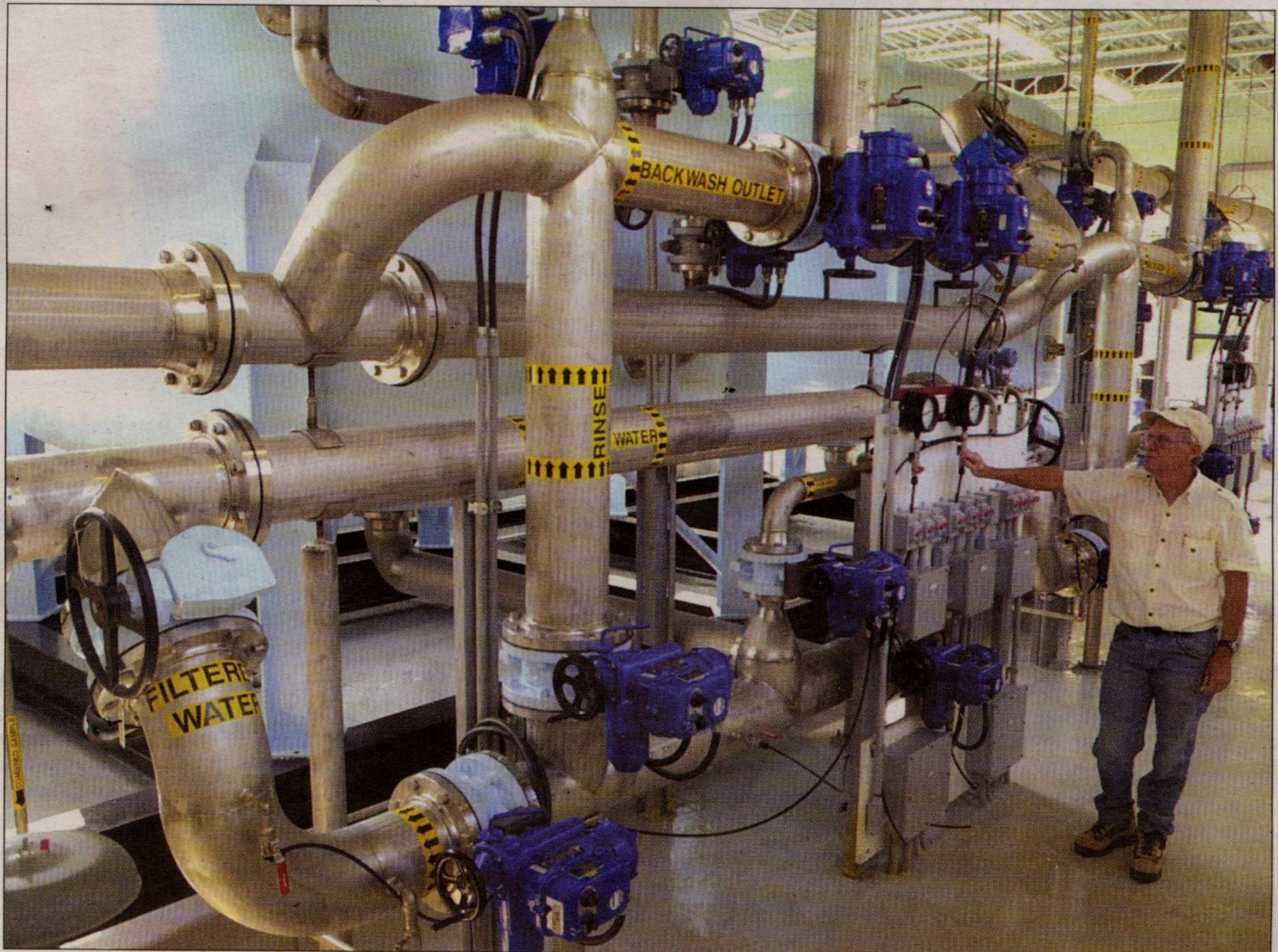
Technician Tom Eisele of Hungerford & Terry Inc. of Clayton, N.J. checks the calibration Tuesday on the filtration system his company installed at the Maple Avenue station. The system, which was put in opera-
