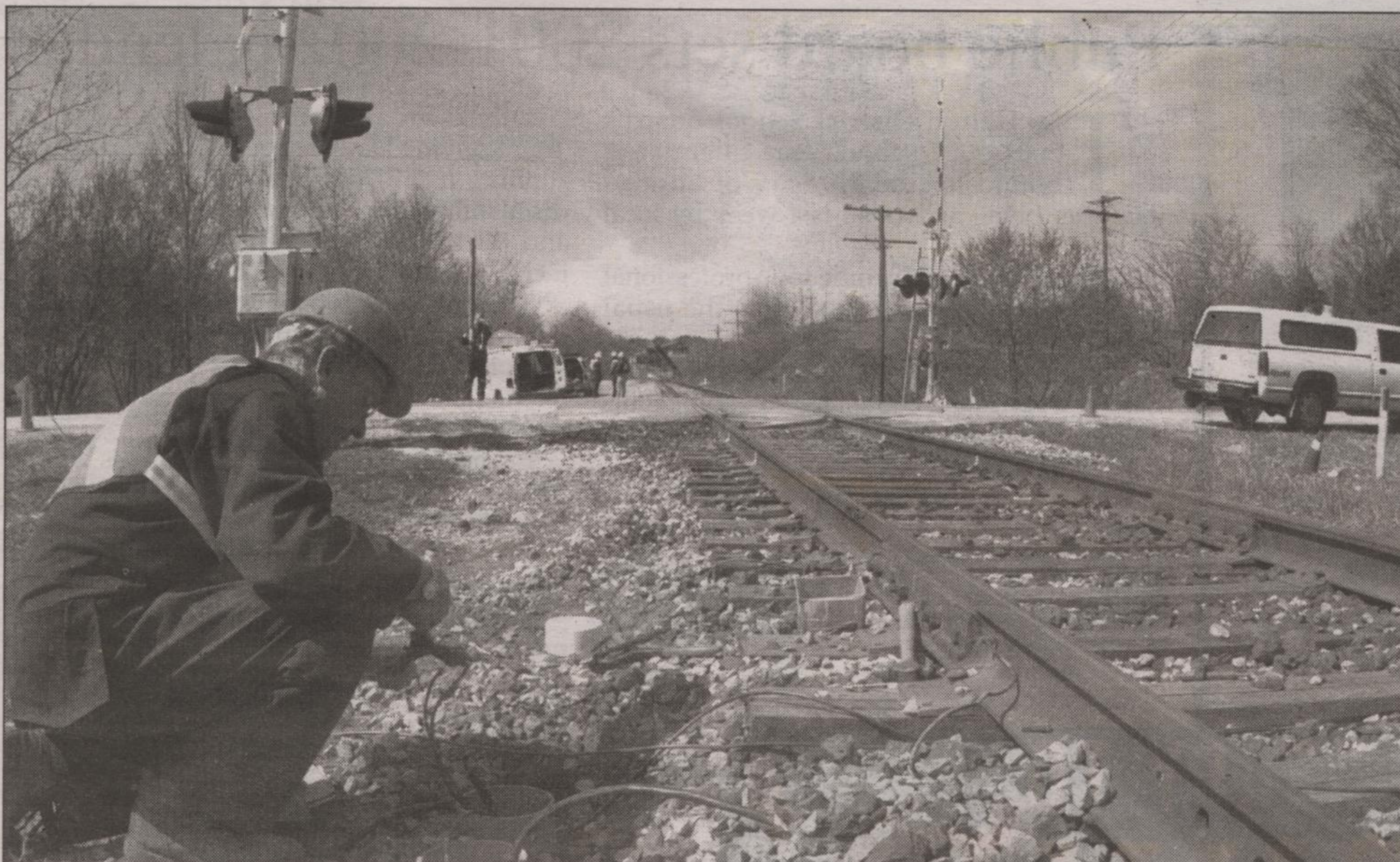
Stu McDonald of AM Signal Systems of Milton finalized the electrical connections on the newly installed signal arms at the Fourth Line railway crossing that has claimed four lives in the past two years. The signals were fully operation late Wednesday afternoon. Photo by Ted Brown
