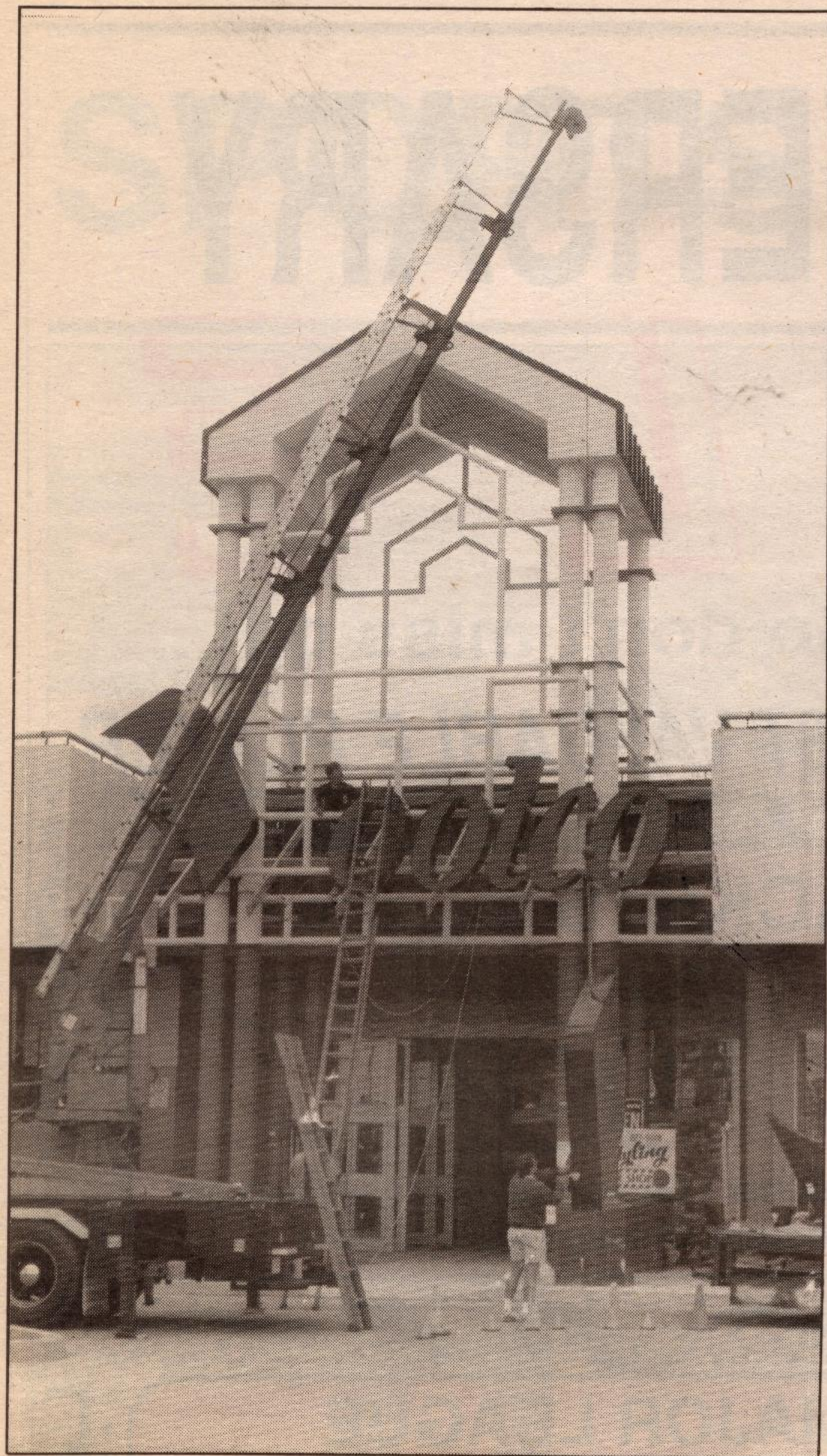
Progress on the Georgetown Market Place mall continued this week as the new sign went up on the front of the building. Woolco is one of the main stores in the converted building. The mall is expected to open before the end of the summer. Photo by Ken Bellamy
