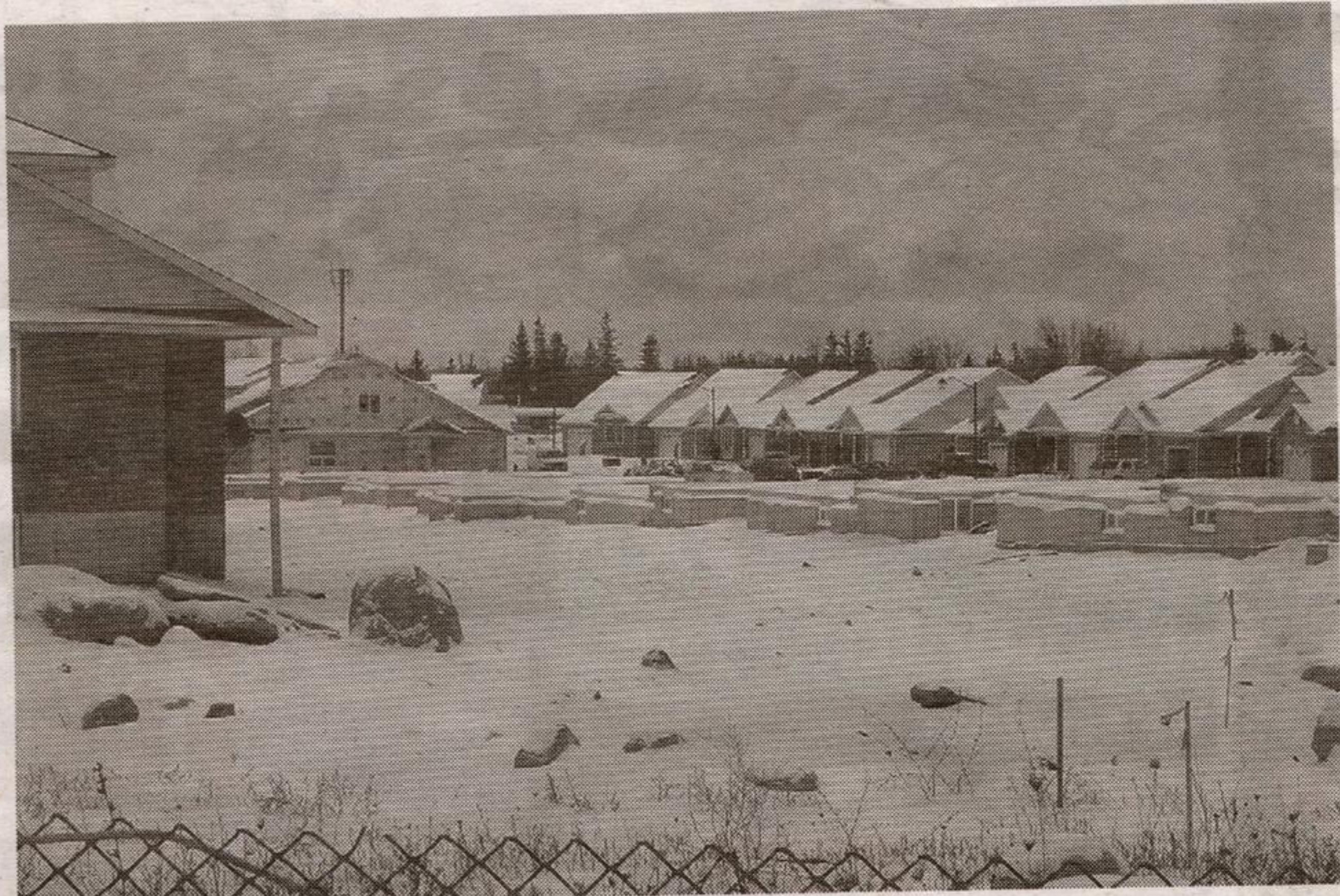
WEATHER OR NOT: Construction continues on new housing on Doctor Moore Drive in the north end of Acton off Wallace St. despite inclement weather.
