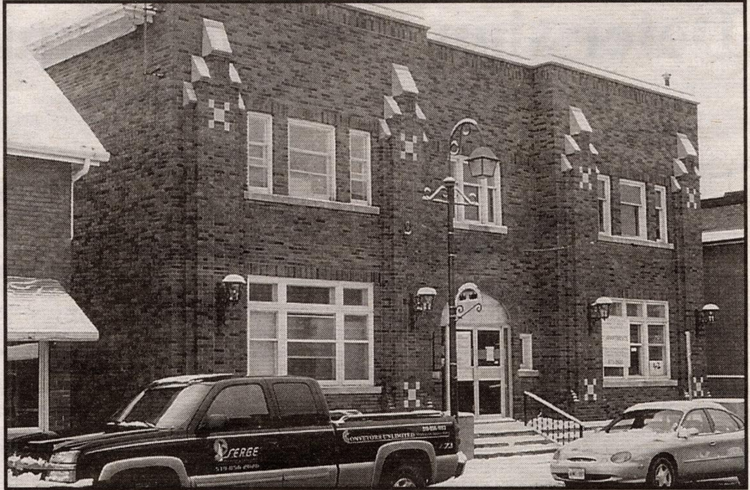
RENOVATING YMCA: Acton's YMCA, a prominent Mill St. landmark since 1934 is undergoing extensive renovations into 'luxury' apartments by a Glen Williams firm.
