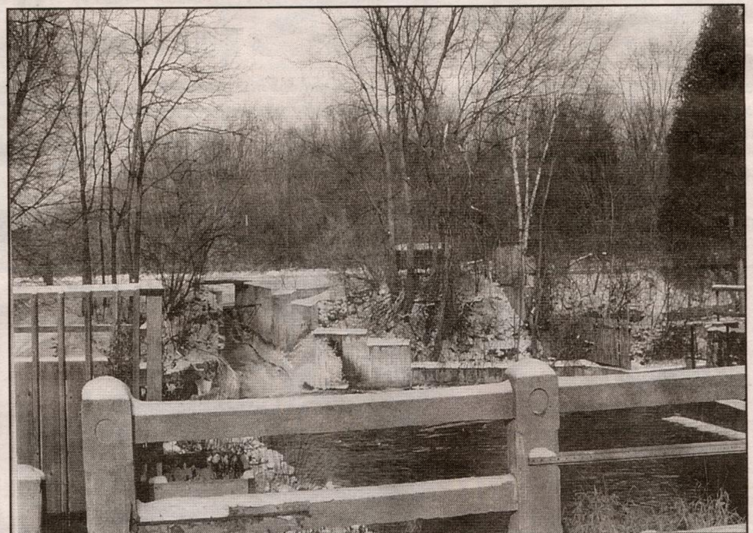
BRIDGE WORK: Service vehicles such as fire trucks, snowplows and school buses can no longer cross the bridge over the Eramosa River in the heart of Eden Mills, shown here. The bridge is deteriorating and a five tonne weight limit has been imposed.
