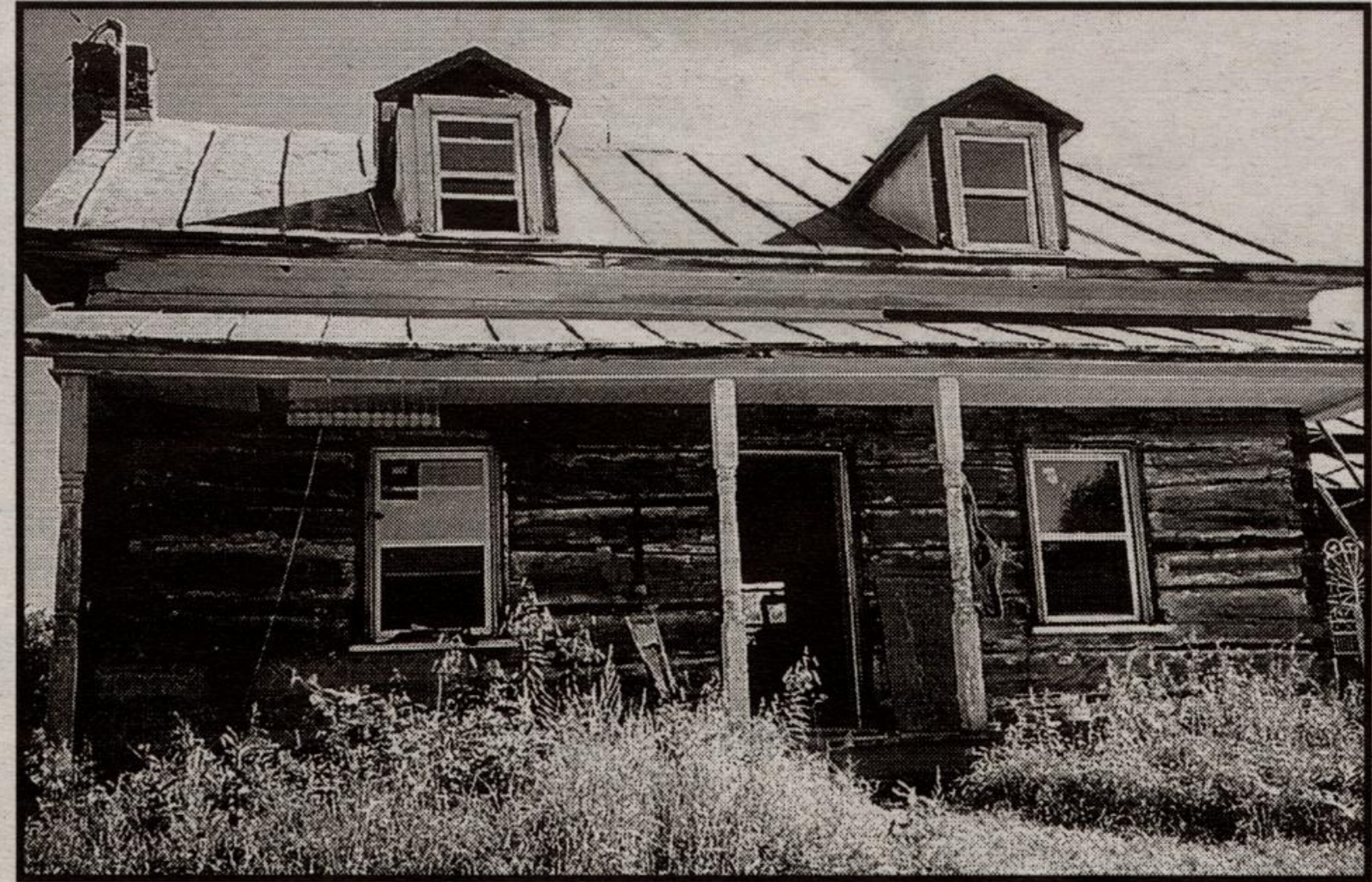
RECYCLING IN THE EXTREME: Farquhar Morrison's log home was built prior to 1850, possibly as early as 1830. It's new owners have gutted the structure to its walls, installed a new furnace and are hard at work turning the antique into a very livable modern home. - Maggie Petrushevsky photo
