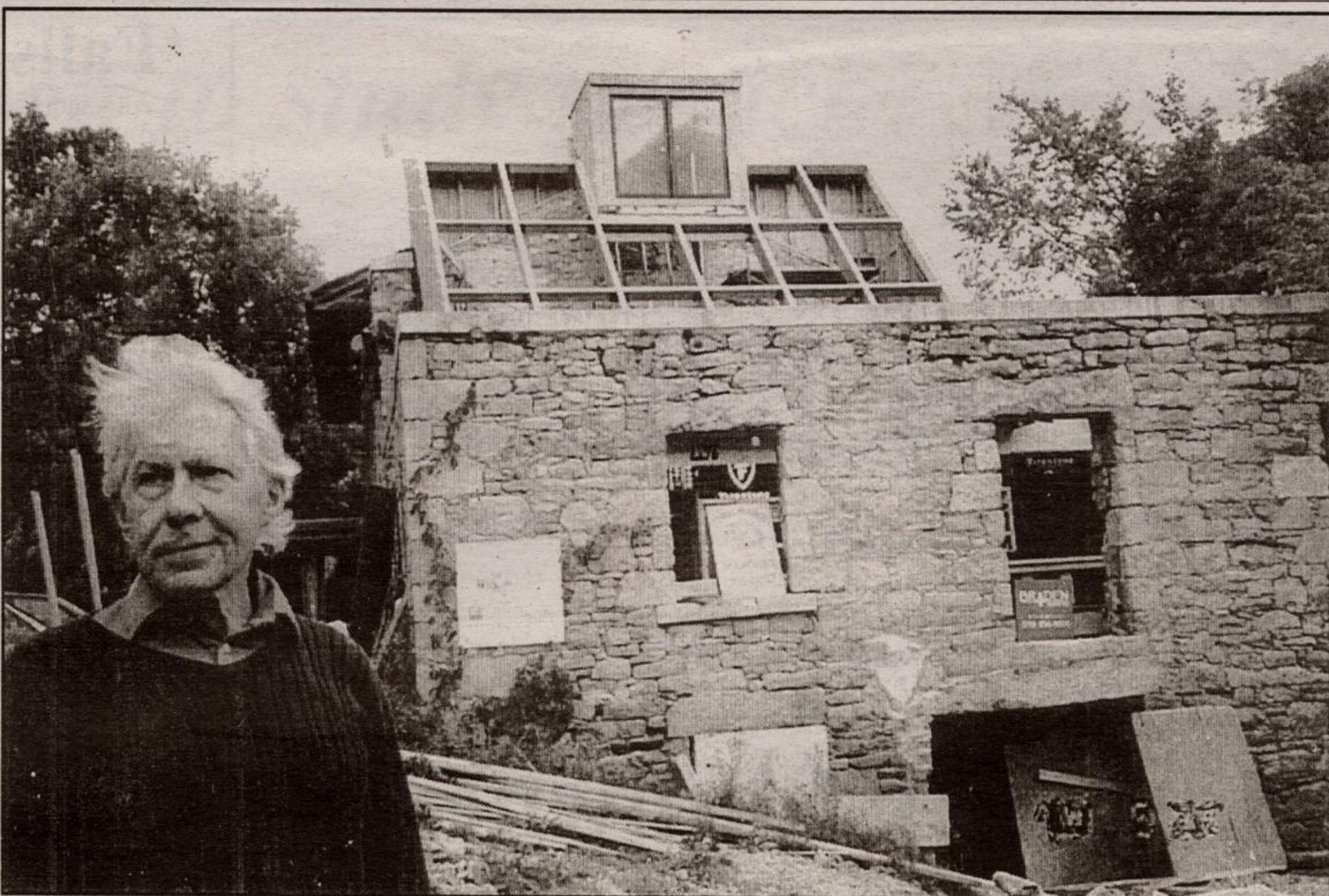
RECYCLING TODAY: Charles Simon is completing renovations to the ruin of the Barden Mill in Eden Mills creating a home, office, studio and guest quarters for himself and his wife. A greenhouse based on solar principles is at the heart of his strategy to use natural systems for the heating, cooling and even some of his electricity. - Maggie Petrushevsky photo
