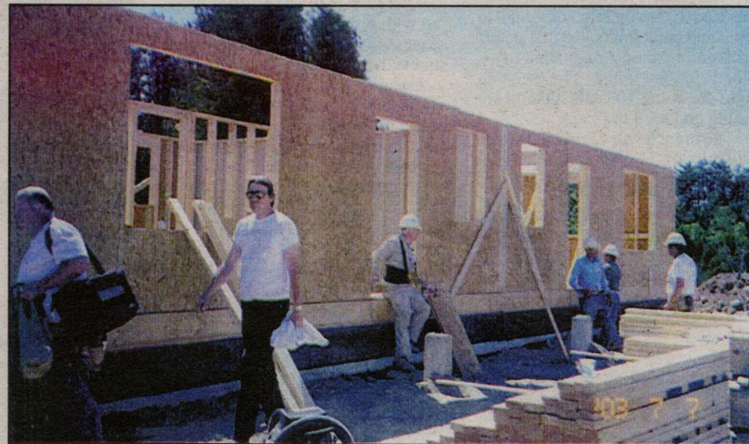
HABITAT FOR HUMANITY: Construction began Monday, July 2, on one of two semis for Habitat for Humanity in Rockwood. When the volunteers called it a day they already had frames up for the first floor of both homes and four walls in what will be finished basements in the units. - Maggie Petrushevsky photo
