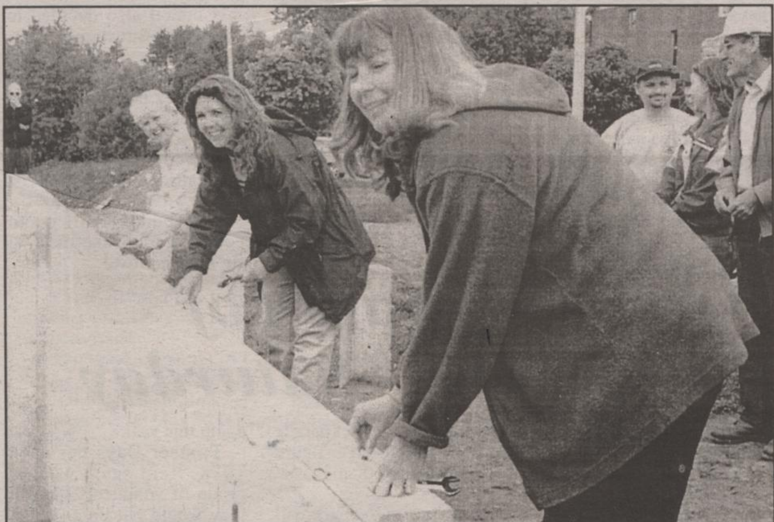
GETTING STARTED: Bobbye Goldenberg, far left, president and CEO of Habitat for Humanity Canada helps Kathy Howard, left and Cynthia Woroch, right, tighten nuts on the first plank to be laid in the construction of their new homes. The women will each own one of the semi-detached homes to be built on the Inkerman site this summer. - Maggie Petrushevsky photo
