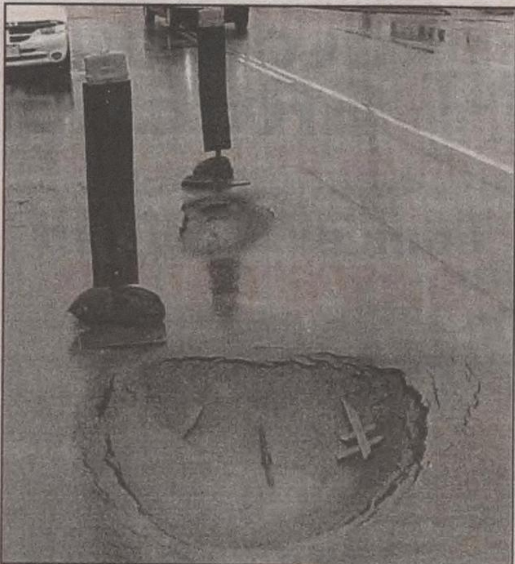
DEFENSIVE DRIVING: These two potholes appeared Sunday evening causing drivers to manoeuvre around them on their Monday commute to and from work. - Ted Tyler photo
