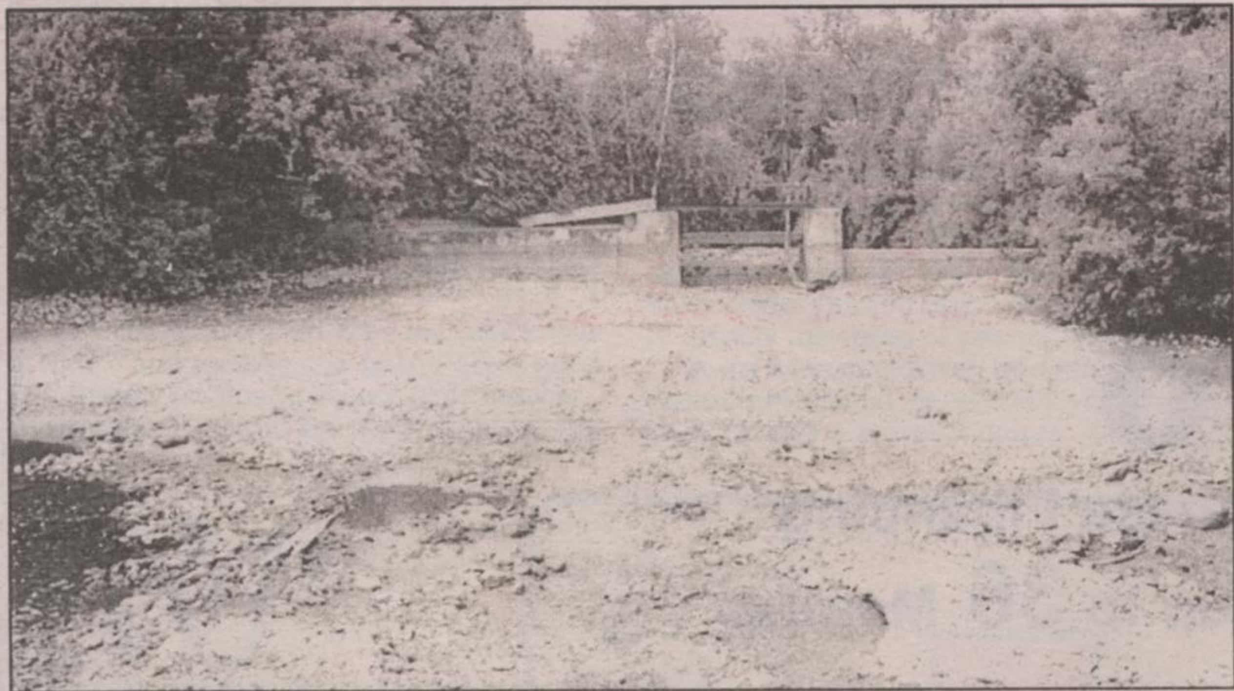
WHERE'D IT GO?: From the highway it looks like the Eramosa River has suddenly found a new channel. Not so, say the owners of the old Rockwood mill. They opened the dam to repair the building. - Frances Niblock photo
