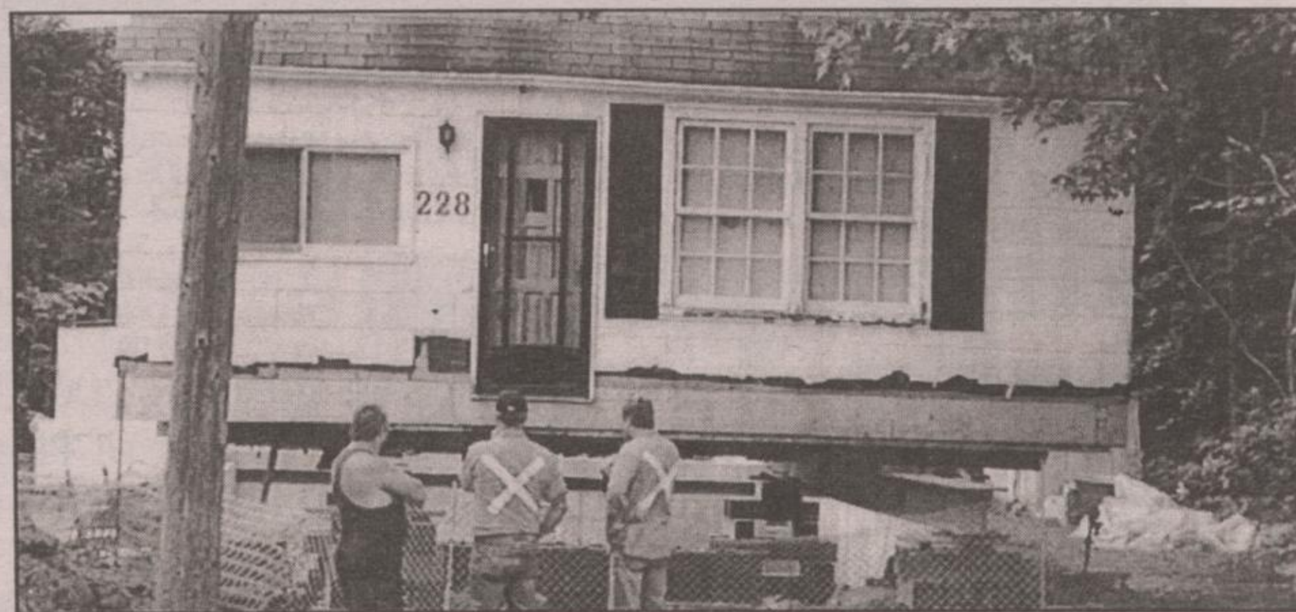
IT'S GROWING: The Chafe family on MacDonald Boulevard like their location so much they decided to put an addition to their home instead of moving. Since the wartime house only had a crawl space rather than a real basement they jacked the house up to put in a full basement to match the basement for their addition. - Maggie Petrushevsky photo
