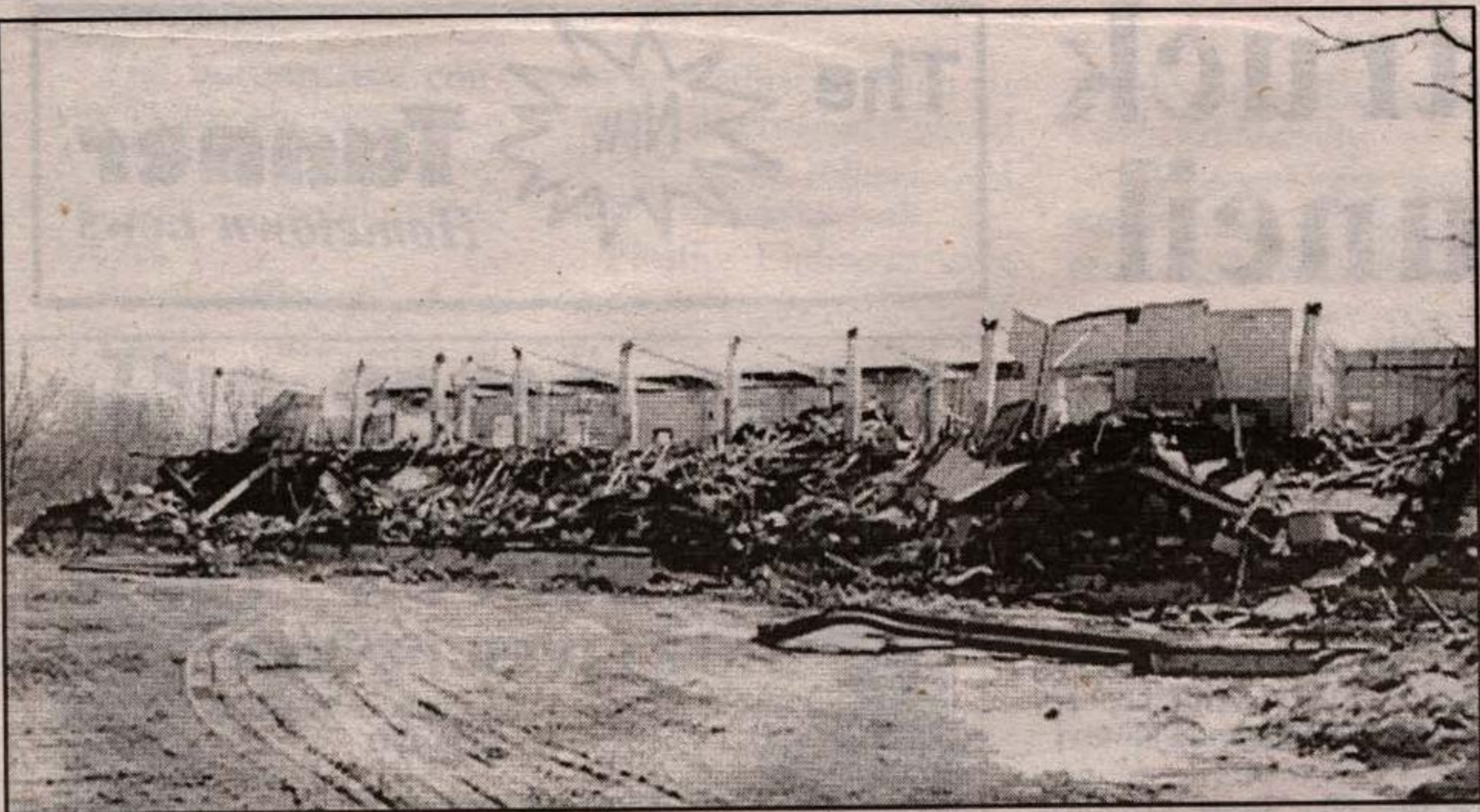
The old AIC (Acton Industrial Centre) building at the former Beardmore property was being torn down last week. - Angela Tyler photo
