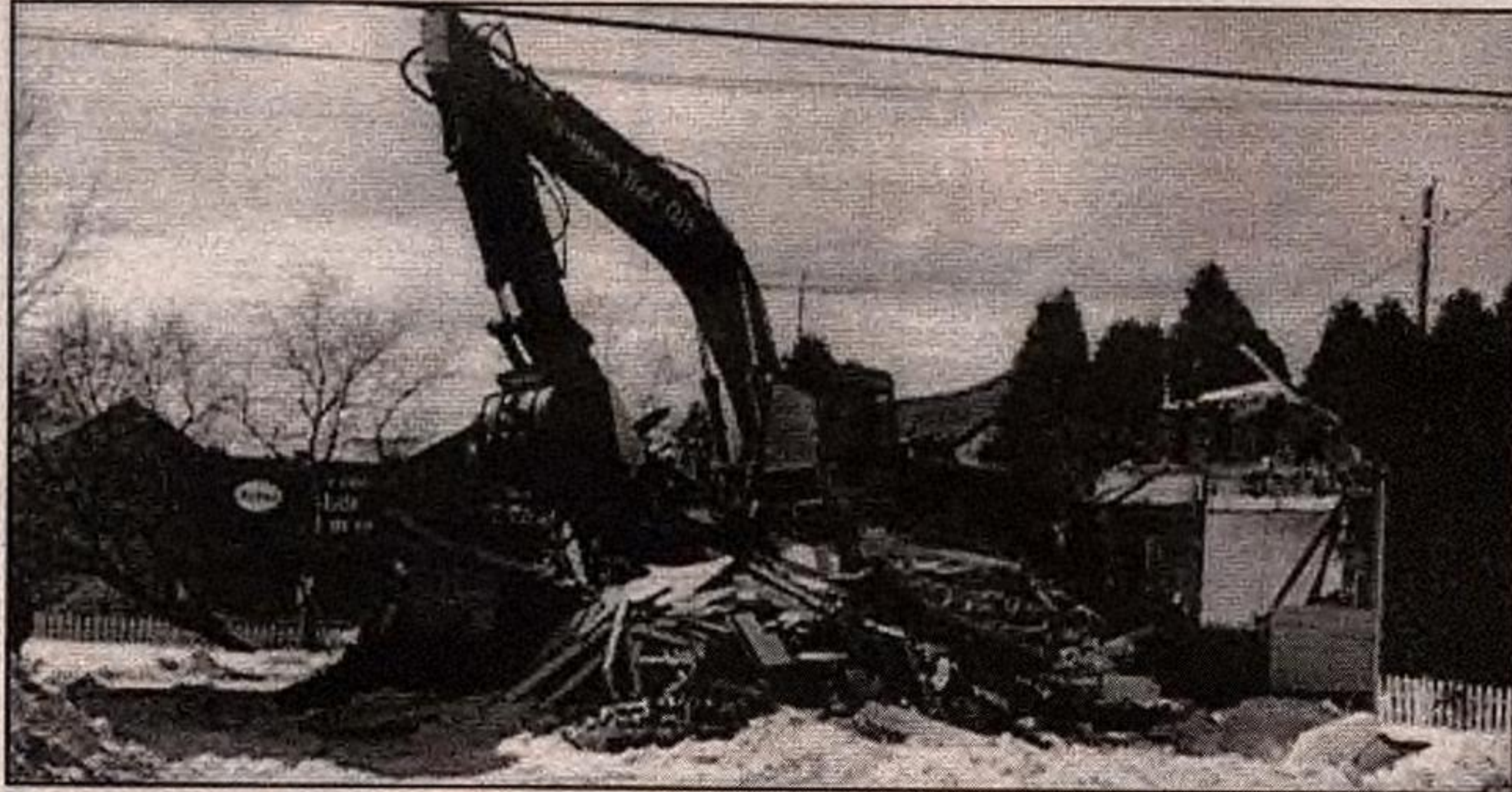
This house on Young Street was completely destroyed a week ago yesterday and the next day there was no trace of it. The house goes back to the 1800s.
