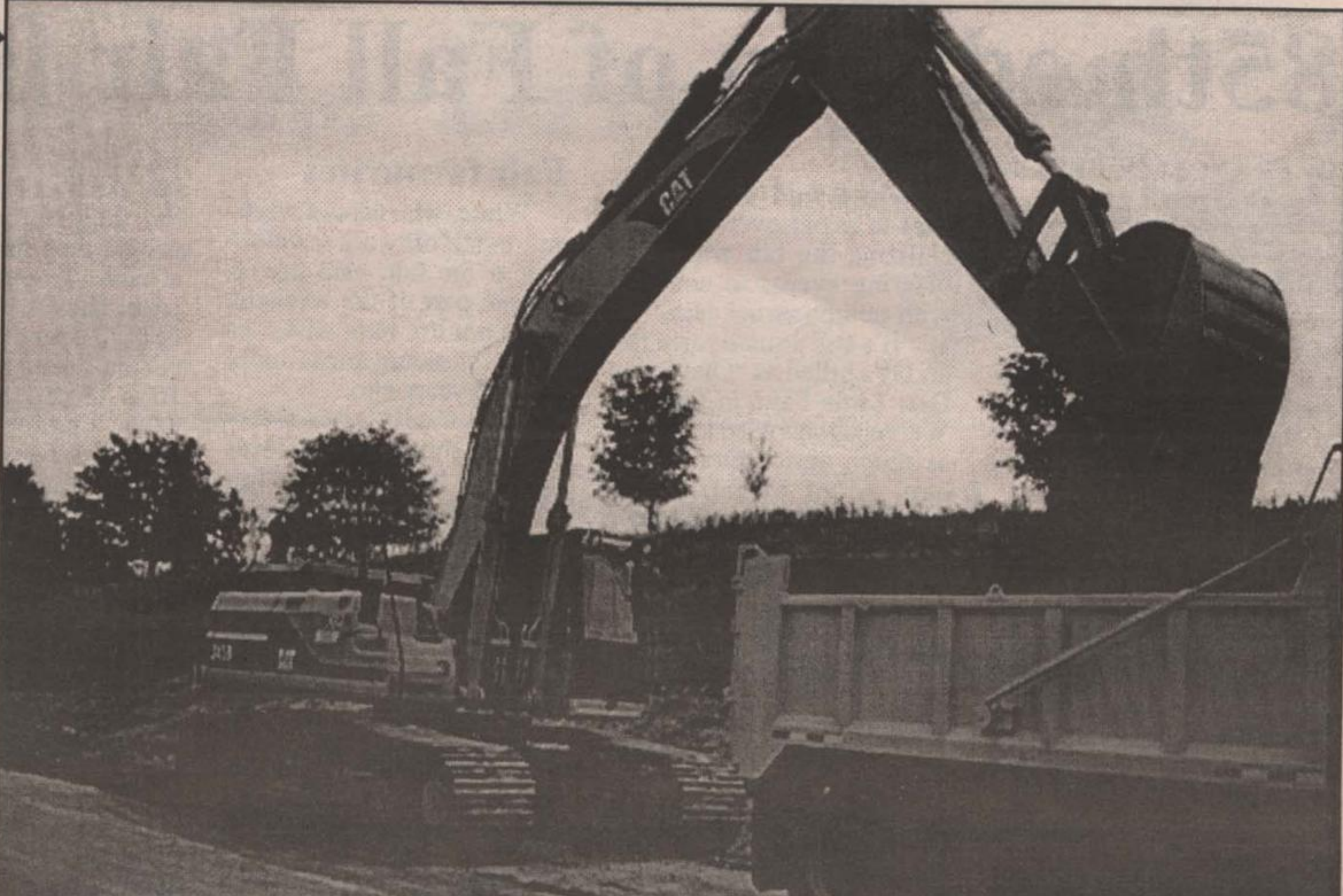
BETTER ROADS: Nellis Construction of Acton has equipment, including this big backhoe, working on improvements to old Highway 25 north of Acton. - Ted Tyler photo
