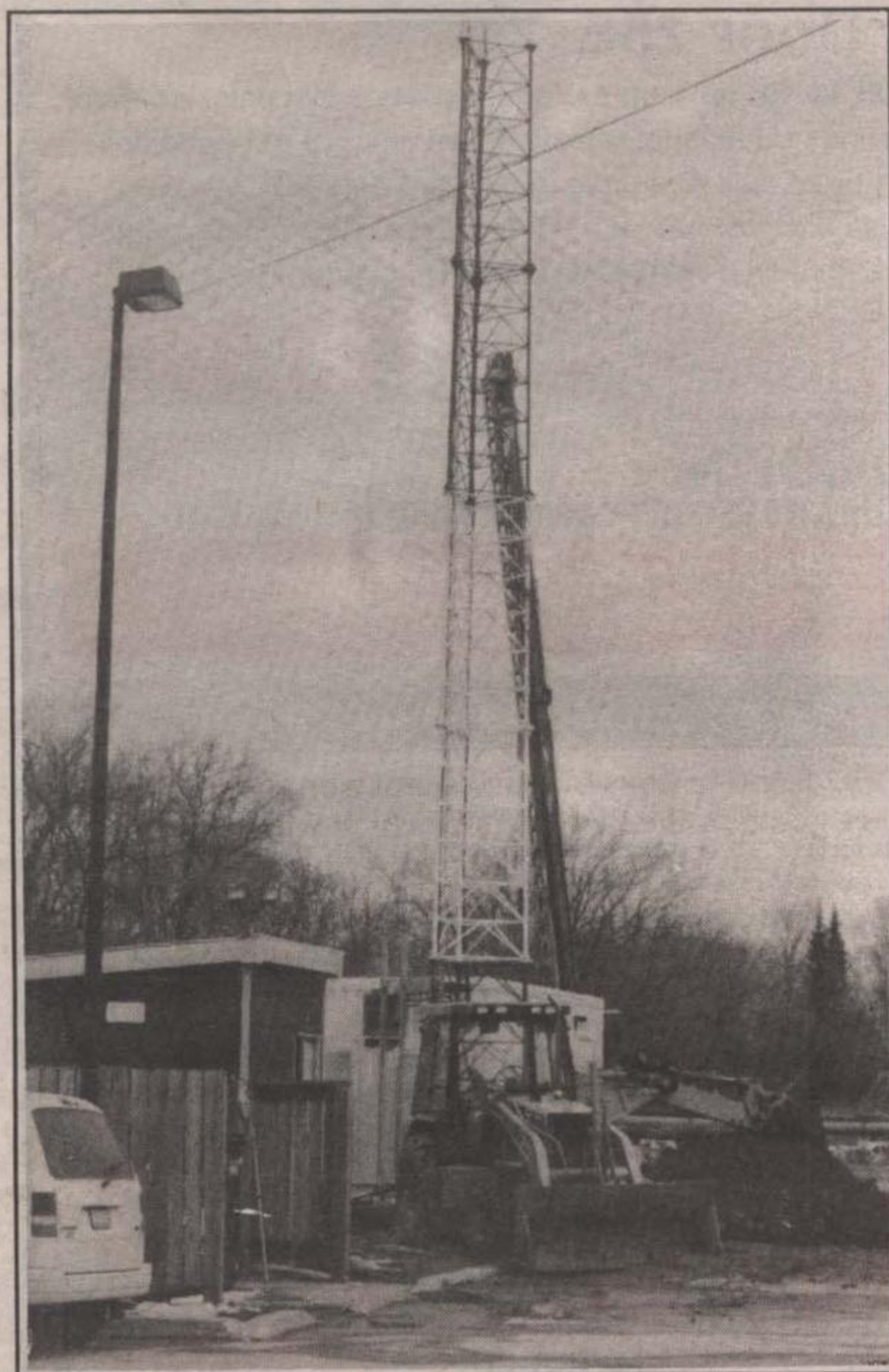
A TOWERING PROJECT: A Bell Mobility construction crew has been hard at work replacing a 40 meter tower behind the Halton Hills Hydro facility on Alice Street. The two-week project is to improve service for cellular phones and PCS service. - Angela Tyler photo
