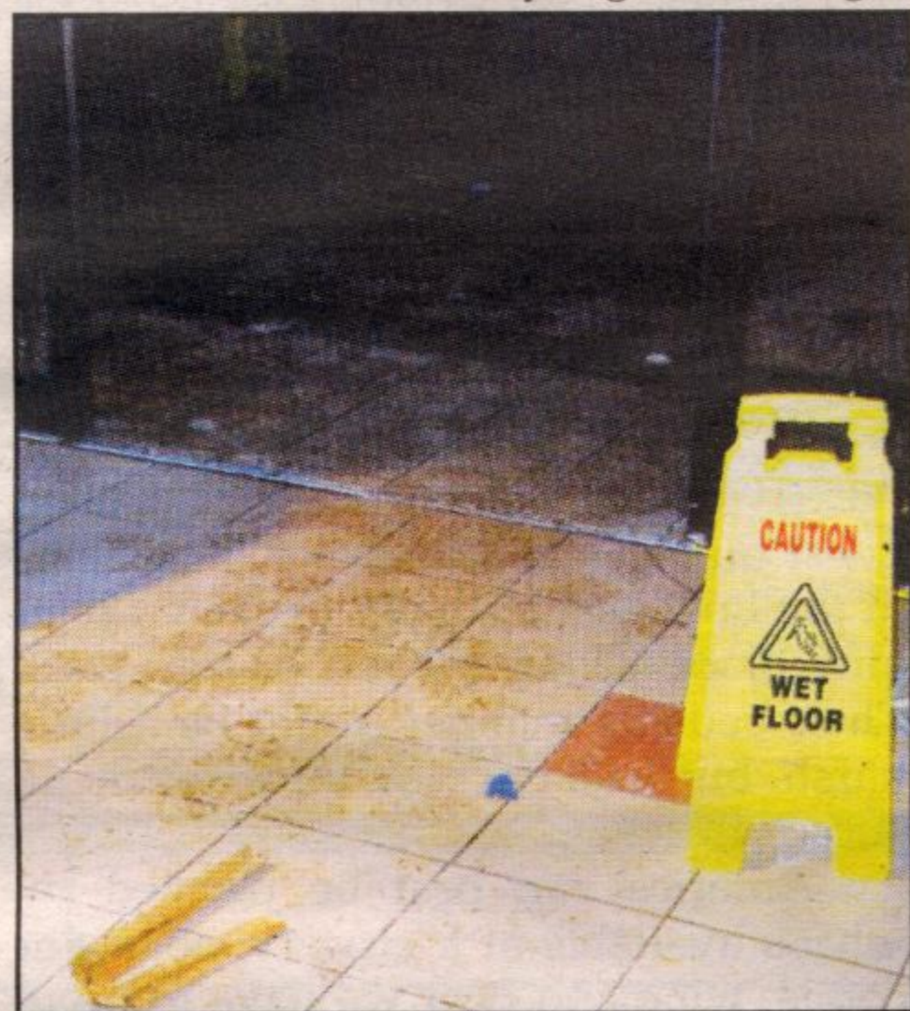
Muddy floors and soaked carpets were just some of the damage done to the Milton Mall when a pipeline burst late Thursday evening.
