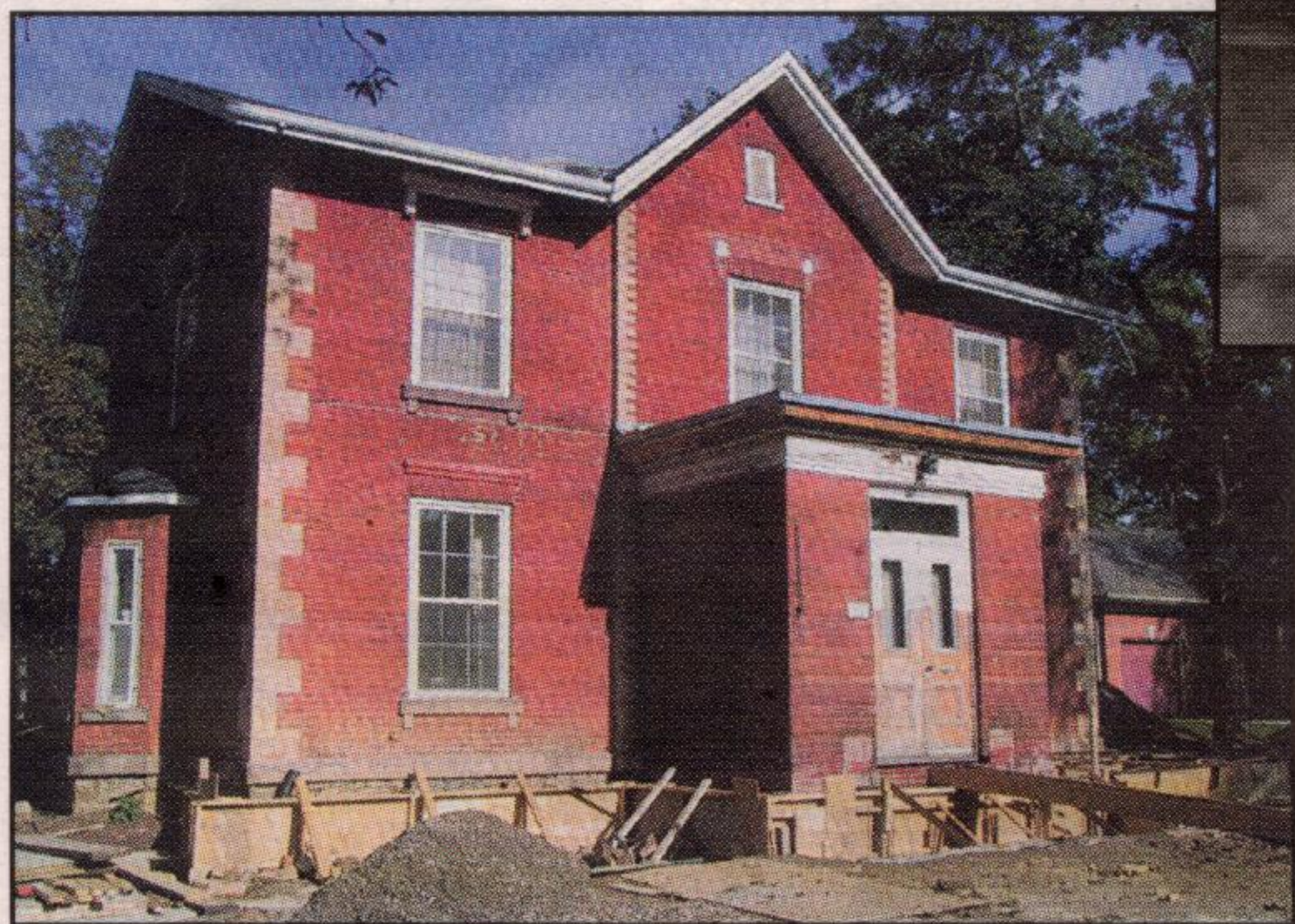
Left: Felsgarth, as it looks today under reconstruction PHOTO BY DEBORAH QUAILE
