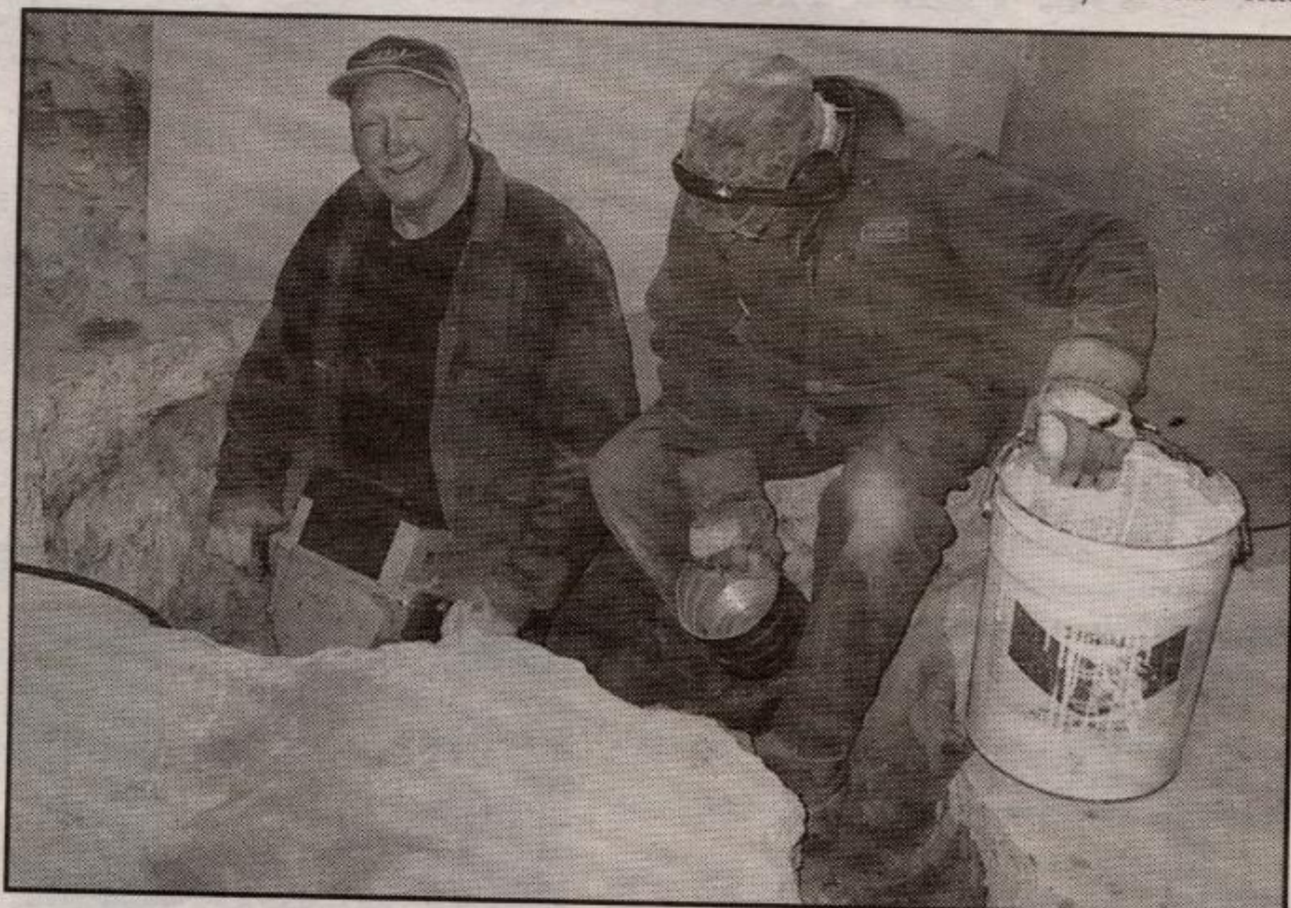
Wally Mayes and John Gmur begin chipping out stone to install new drains for the wheelchair accessible washroom.
