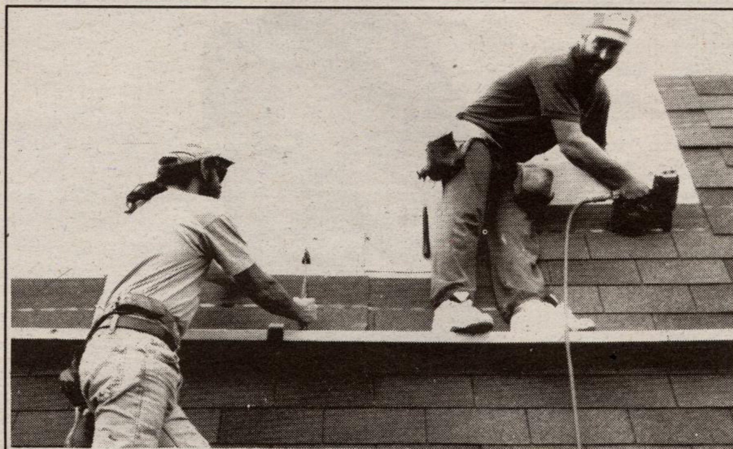
Peter Beaton, owner of Beaton Roofing with foreman Keith Pettliere working on The Teak Barn.
