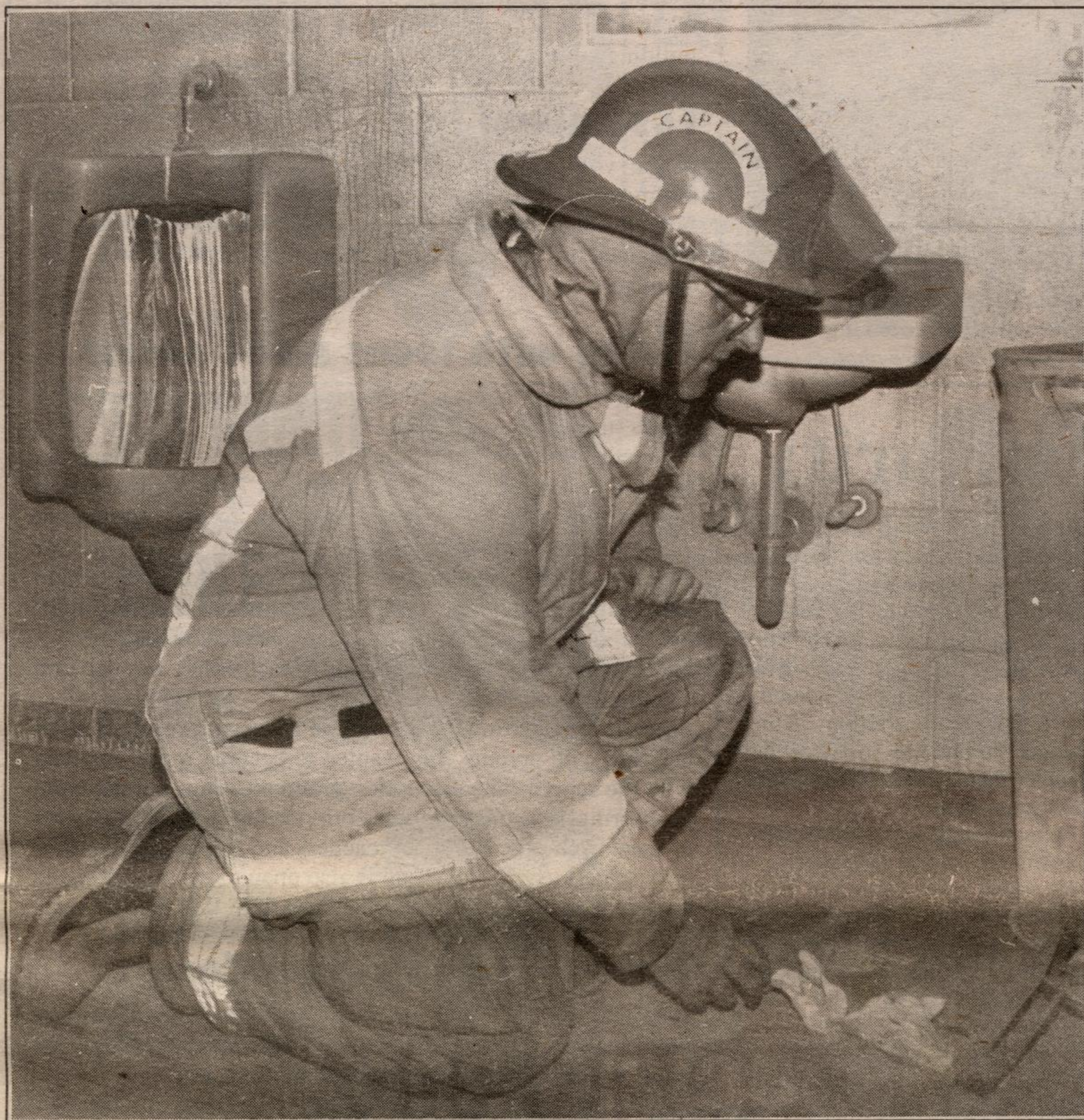
WASHROOM FIRE: Captain Doug Andrews of the Halton Hills Fire Department inspects what is left of a paper towel, which caught fire in a lower level boys' washroom at Acton High last Wednesday. The fire is believed to have caused $2,000 damage. See story on Page 4. (Doug Harrison photo)
