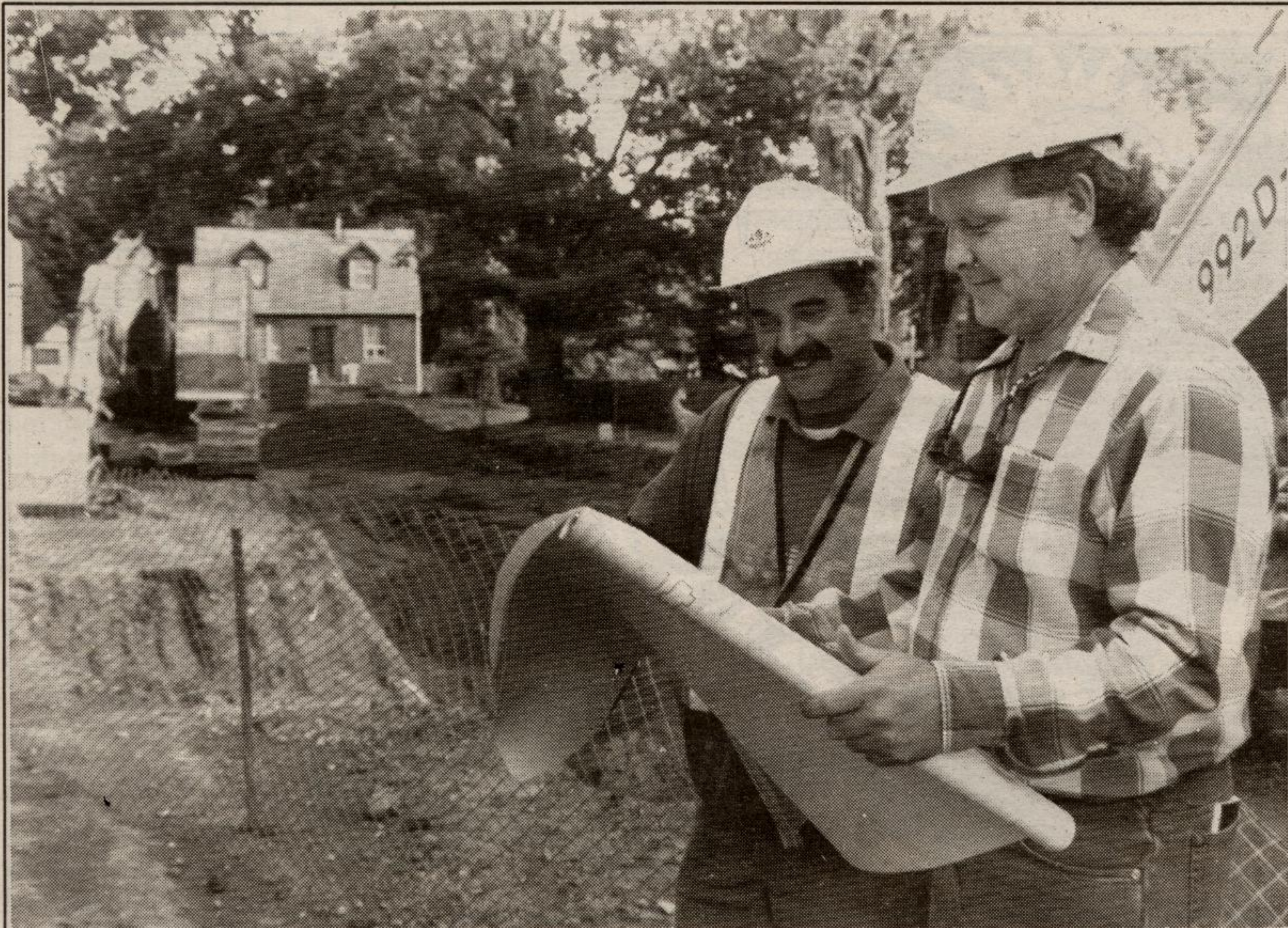
ROAD WORK! Worker Tony Delnero, left, and Halton Region's Brent Hoey look over the plans for construction on Park Avenue Thursday afternoon. The project includes work on the neighbourhood's water main, and a storm sewer will be constructed. The federal infrastructure program provided funding for the work, which won't be finished for a couple of months. (Paul Nolan photo)
